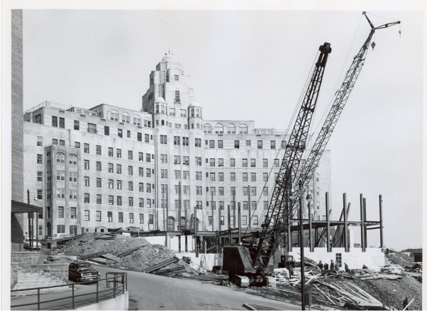
Figure 4: Construction is underway on the south wing expansion of the Saint John General Hospital. Photographer: Climo Studios. 1957. Reproduced with permission of the New Brunswick Museum (Accession # Acme-F4-3).
