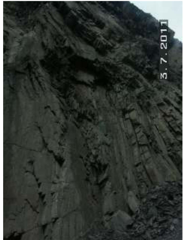
Fig. 1 Buckling failure of rock bedded slope in K745
