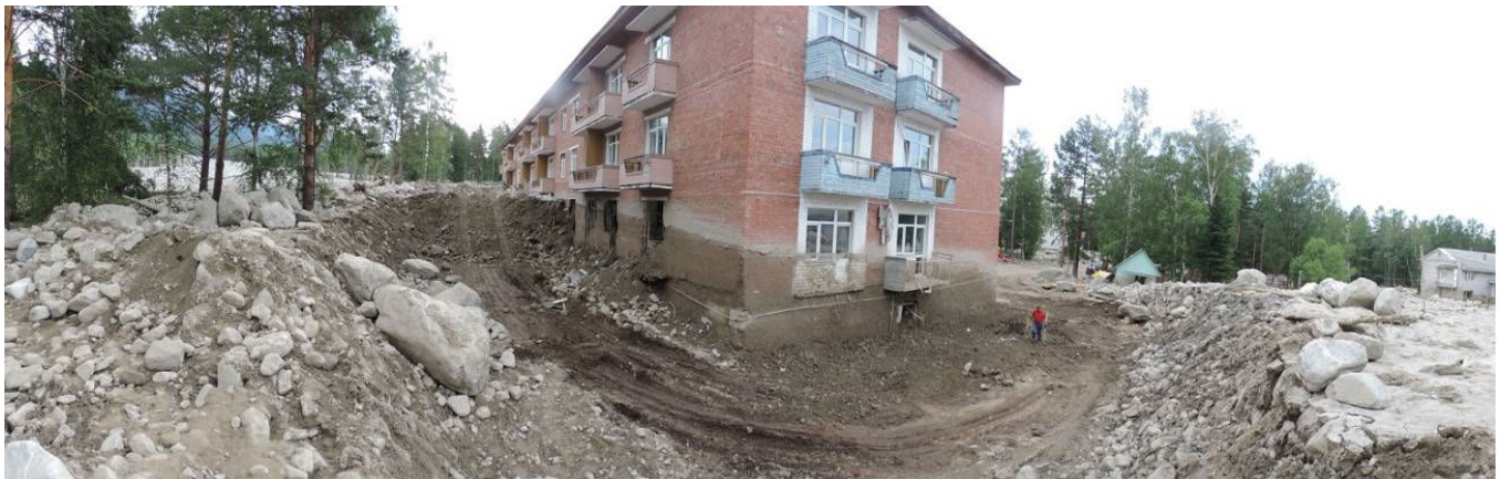
Figure 9. Building of medical rehabilitation center “Sagaan Dali” obstructed with debris flow deposits descended along the river Vtoraja Shikhtolaika. Picture of July 9, 2014 (point 740 – 51°54'29.0", 102°26'45.2")
