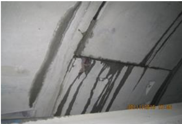
Figure 6. Slurry leakage between segments
