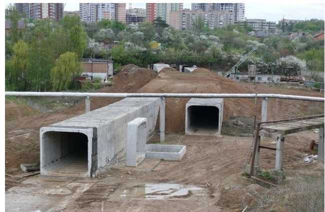
Figure 10. Construction of tunnels through the Oleksiivska ravine between the 23 Serpnia and Oleksiivska stations. Photo source: KHARKIV Today, https://ua.news/ru/yevrosoyuz-profinansuyebudivnitstvo-harkivskogo-metro/
