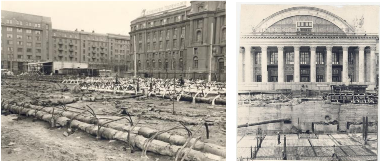
Figure 5. System for freezing quicksands during construction of the Pivdennyi Vokzal metro station in Kharkiv (picture from 1971). Photo source: http://www.mirmetro.net/kharkiv/cruise/01/11_pivdenny_vokzal
