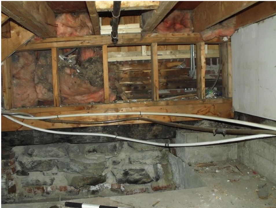
Plate 5 – An open space below the main staircase, accessible only from the basement through a niche or recess in the eastern wall. Looking east.
