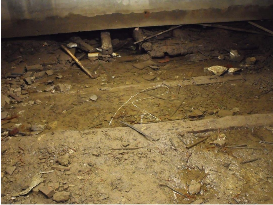
Plate 1 – Tidewater seeping into the basement, approximately 20 minutes before a moderate high tide.
