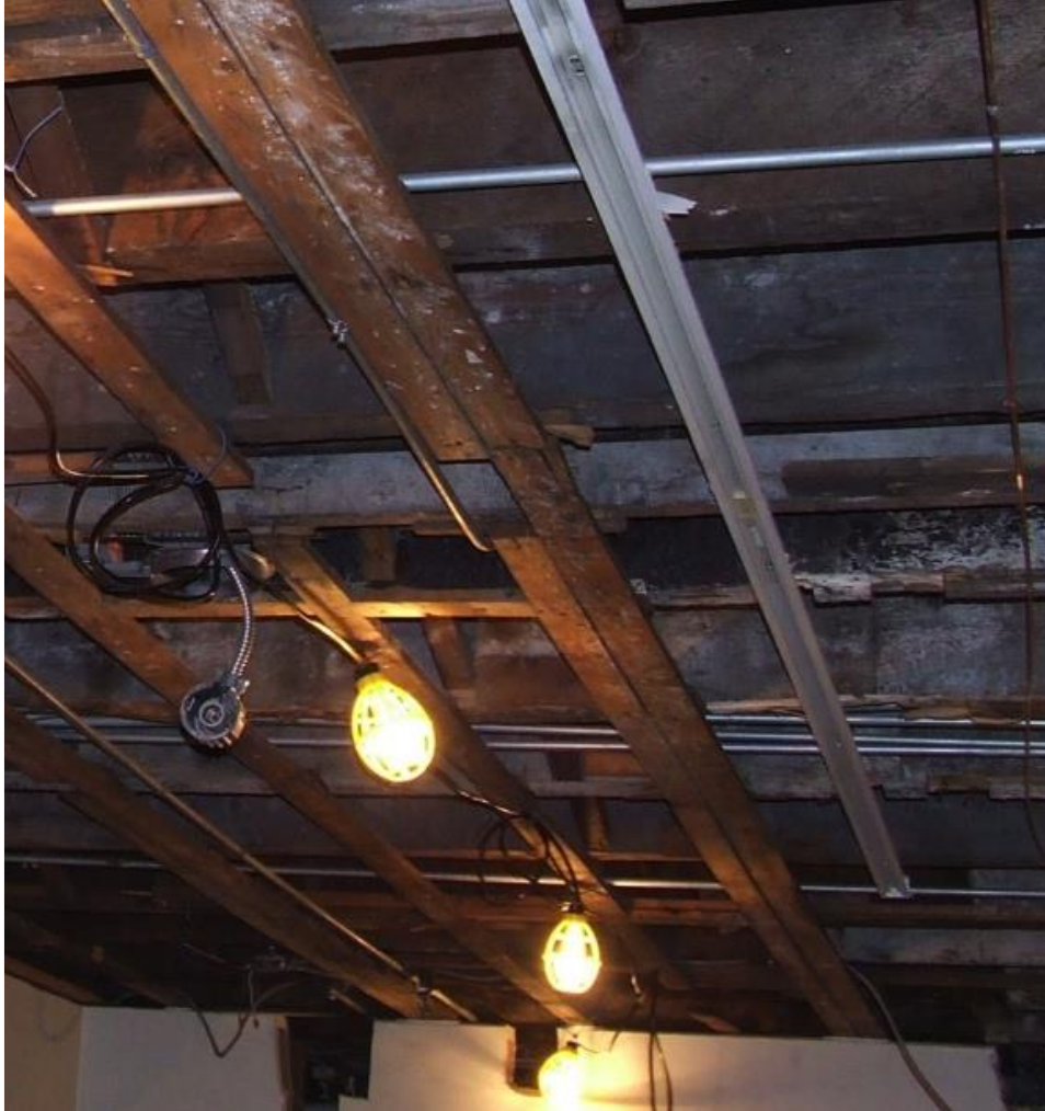
Plate 18 – Charred timbers above the visible storage area behind the Robertson Store reconstruction. Image courtesy Dan Conlin, Maritime Museum of the Atlantic.
