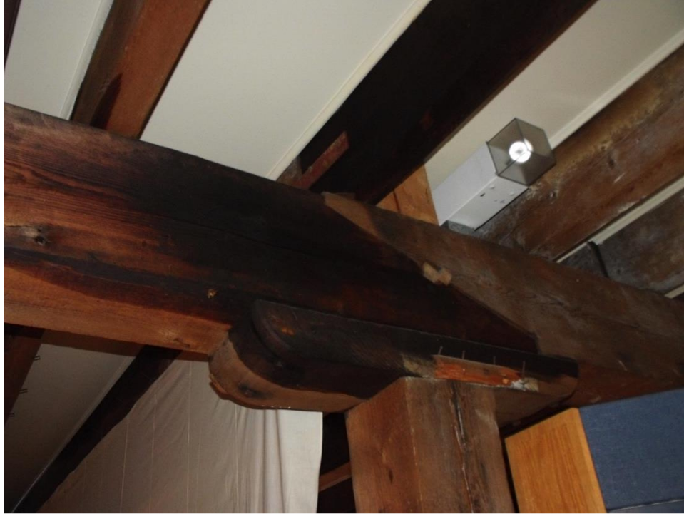
Plate 40 – Oil-saturated wood on the southern running beam, looking northeast.
