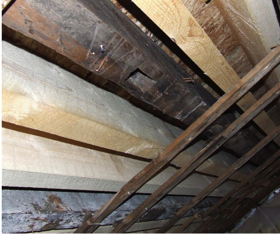
Plate 31 – A reused joist in the ceiling of the second floor meeting room. Note also the new reinforcement beams and the heavy charring on the old beam at the bottom of the photo. Image courtesy Dan Conlin, Maritime Museum of the Atlantic.
