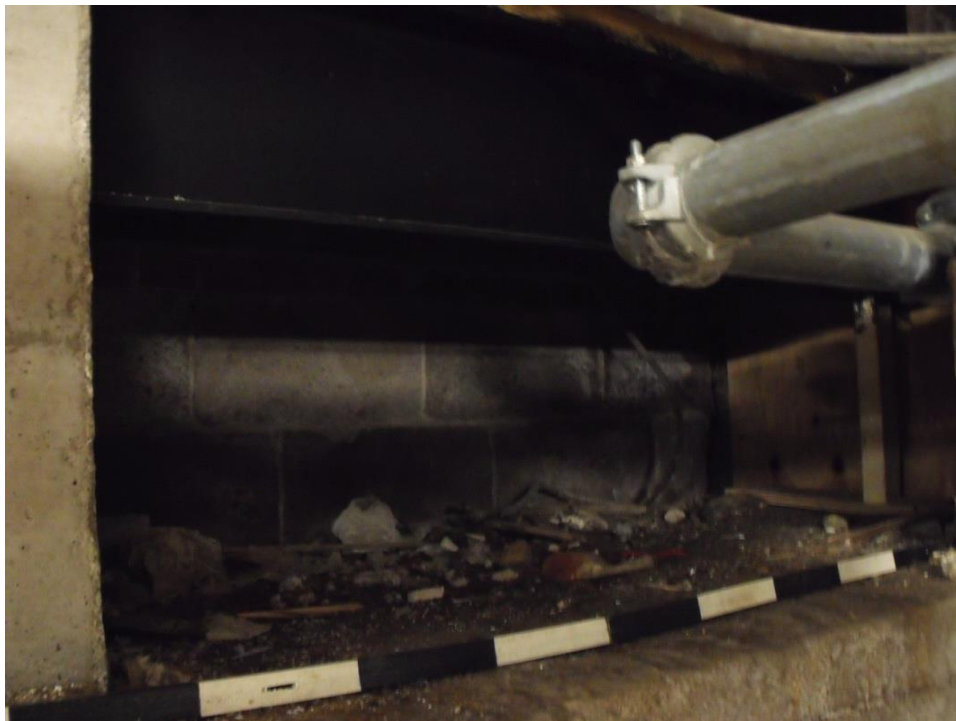
Plate 8 – The southern recess in the east wall, showing modern cinderblock at the back.
