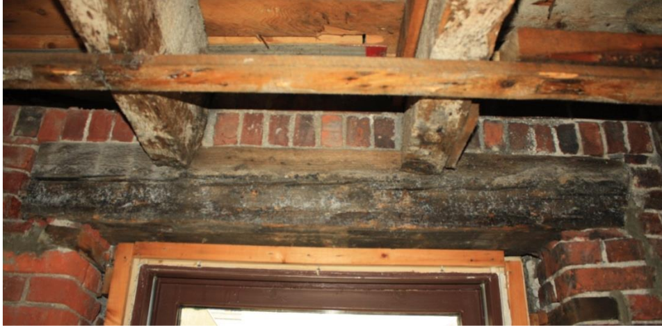
Plate 32 – A heavily charred lintel above a west-facing window in the second floor meeting room. Image courtesy Dan Conlin, Maritime Museum of the Atlantic.
