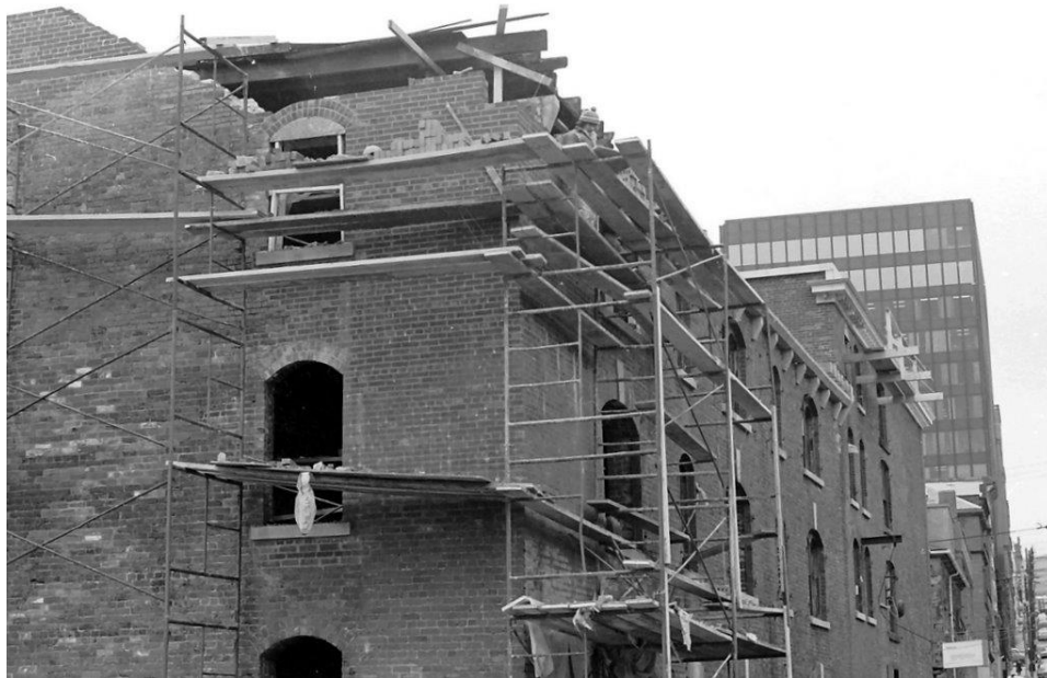
Plate 69 – The eastern and northern faces of the building, showing partial disassembly of the third floor brick and northern cornice. Image courtesy Stephen Archibald.
