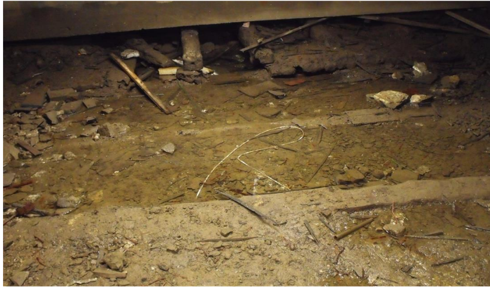
Plate 9 – Half-buried joists in the mud and dirt floor of the basement. Note the remains of planks over them at the top of the frame, below the concrete beam. Looking south.
