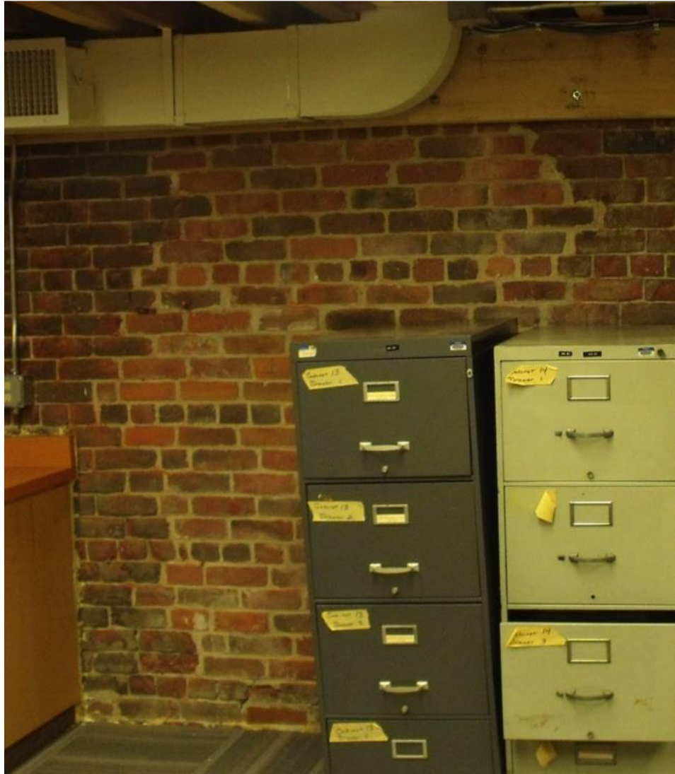
Plate 56 – A blocked window is evidenced on the western side only by the cleanliness of the brick and the new mortar.
