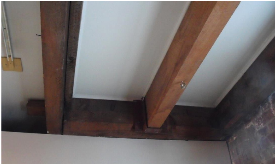
Plate 38 – An extra crosspiece and a new joist near the southeast corner suggests the former presence of a staircase. Looking north.
