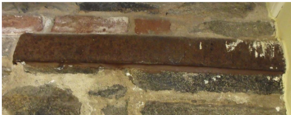
Plate 50 – A 32" iron strap extending along the south wall from the southwest corner, likely helping to secure the brick façade to the main building.
