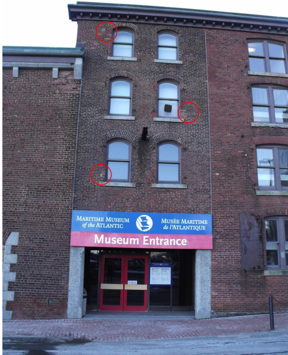
Plate 67 – The infilled section on the building’s north face. Note missing brackets for iron shutters at repair points (red).
