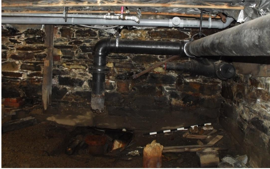
Plate 13 – The storm drain at the northern wall, looking west.
