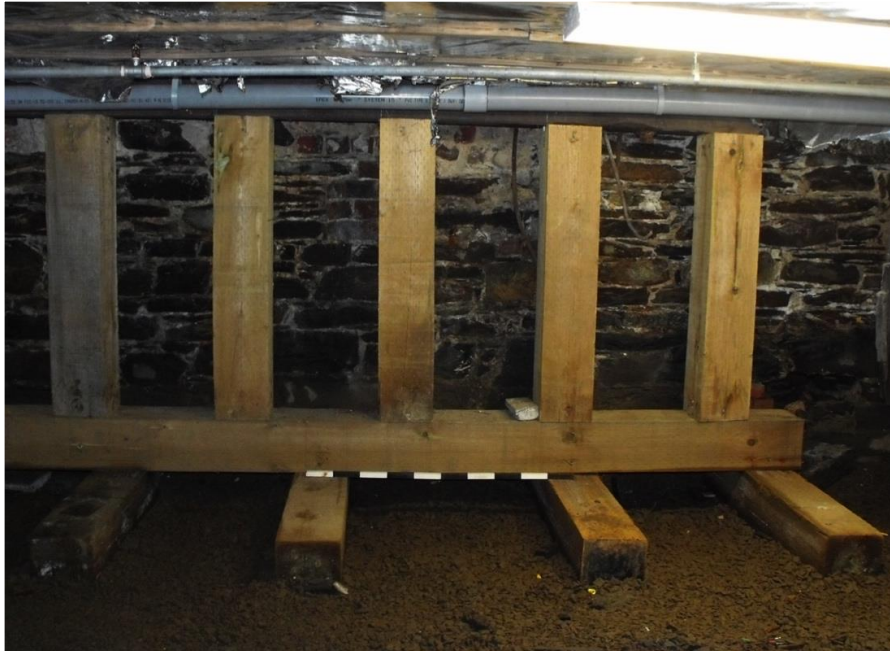
Plate 14 – Late twentieth century wooden supports below the main shop entrance on the west wall.
