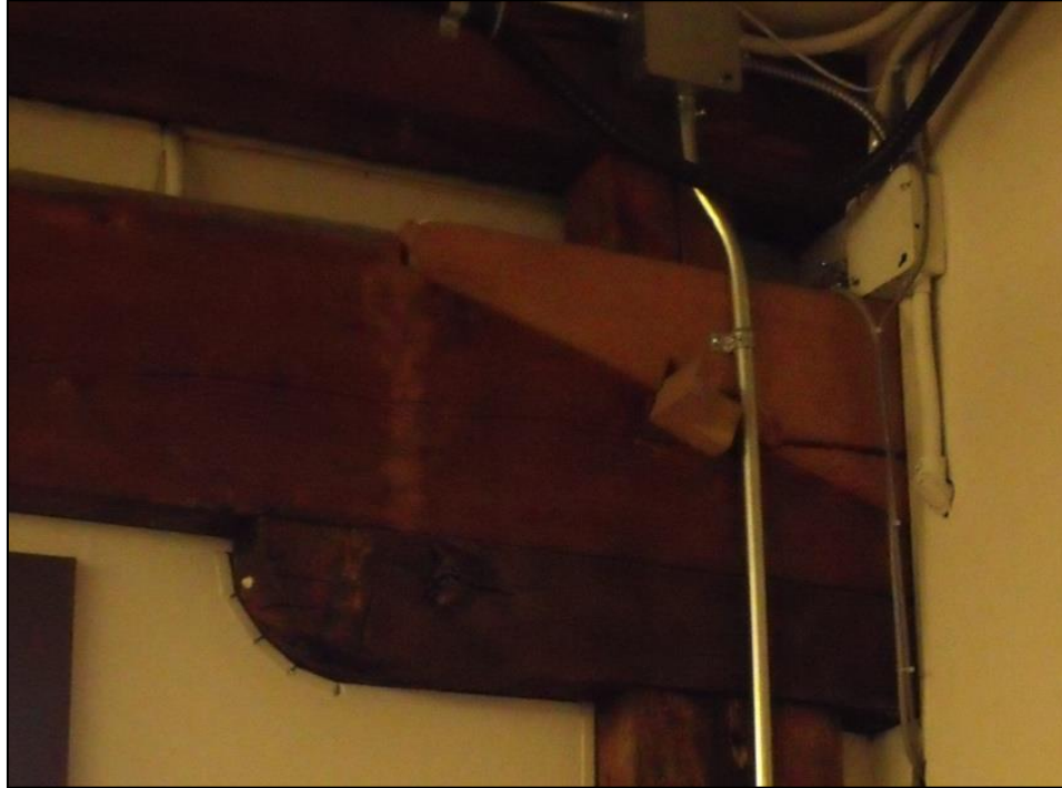
Plate 60 – The exposed eastern scarf joint in the northeast corner, showing a replaced (lighter) section of the beam.
