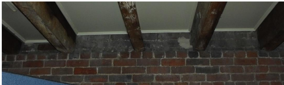
Plate 42 – The south wall at the top of the second floor, showing a step back by one brick width to allow the floor joists to rest above it.
