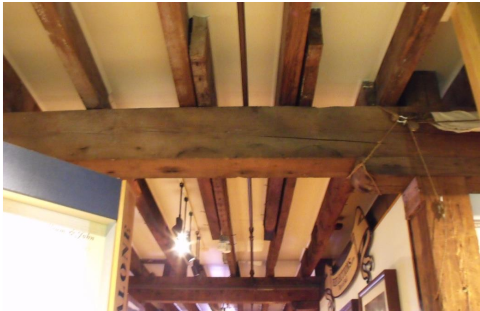
Plate 39 – Modified and truncated beams near the middle of the warehouse. Top and middle: Looking east. Bottom: Looking north.
