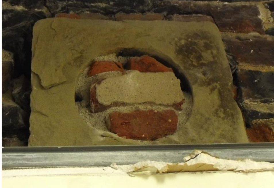
Plate 20 – A blocked sandstone thimble above the drywall sheet in the electrical room.
