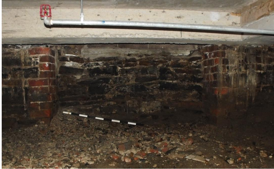
Plate 3 – Mineral and salt build-up over two of the brick quoins that form almost all of the corners in the basement. East wall, north-east corner.
