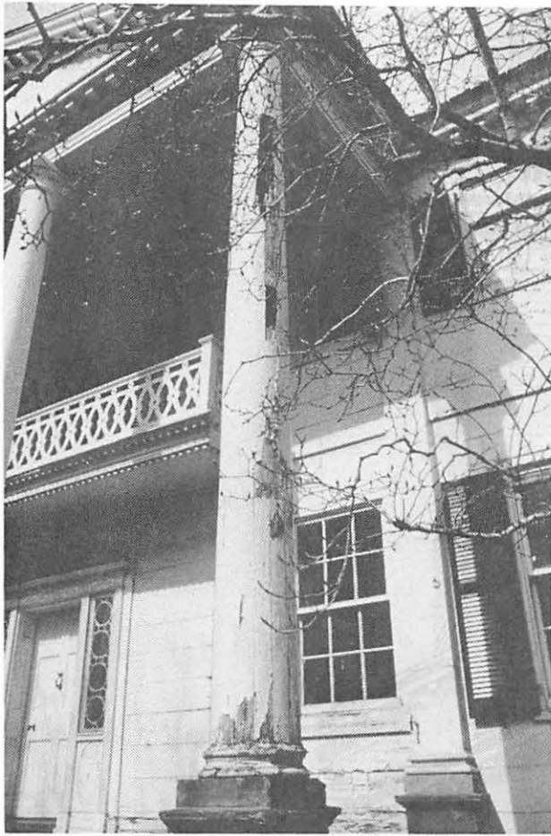
Illus. 52 Rotting wooden column of Jumel house, before restoration by the City of New York. Penney photo. See Penney, p.38.
