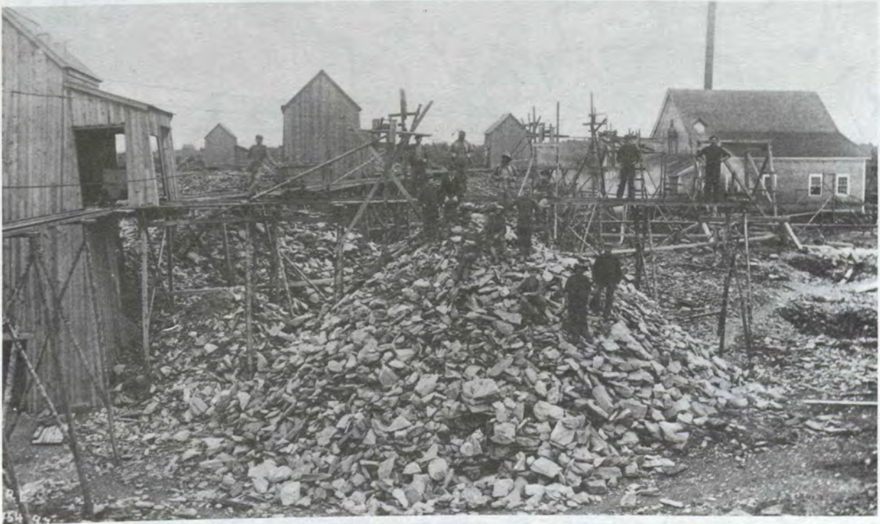
ILLUS. 22 - Shaft structures. New Glasgow Gold Mining Company, 1897. PAC 51444. Tramways connect to mill building at right.
