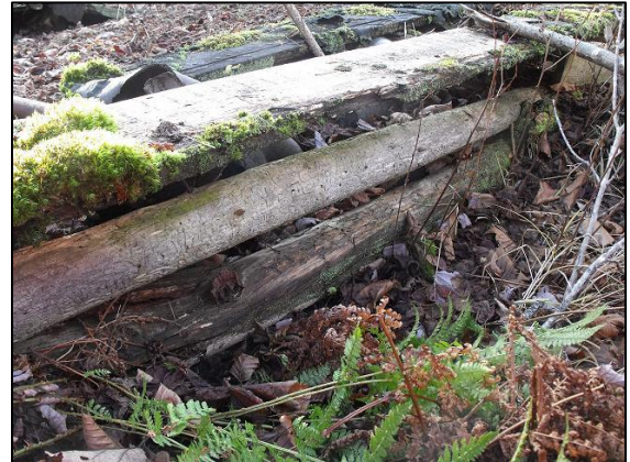
Plate 1: Wooden sill and plank construction of cabin, looking southwest. Note the wooden sills are placed directly on the ground.
