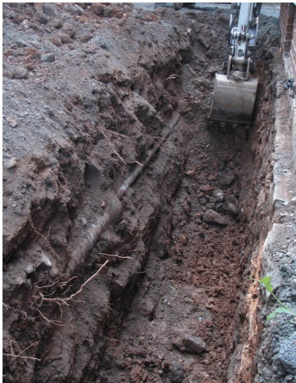
Plate 2 - Pipe in left profile of trench on eastern (driveway) side of house.
