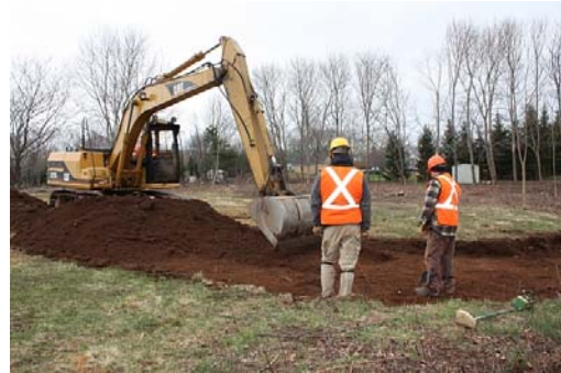
Figure 1 – Mechanical removal of the topsoil to expose archaeological features. (Photo by Jonathan Fowler)
