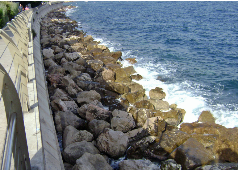
Fig 3 Section of an armoured seawall at the foot of a steep hillside that faces the Mediterranean Sea in the lower city area of Monaco. The rock armour apron is intended to prevent the seawall's foundation from being undermined by wave erosion during intense storms (Photograph by author).
