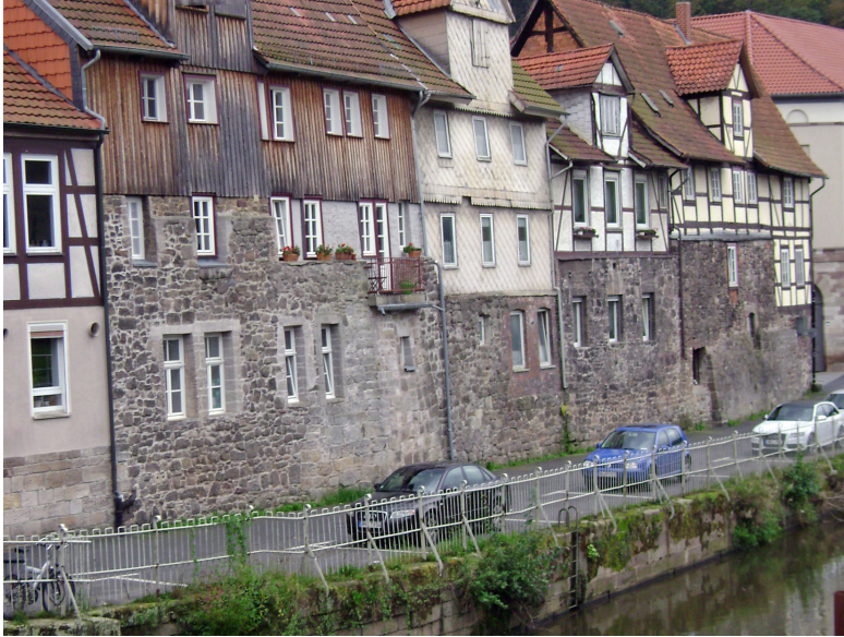
Fig 2 Photograph of some 15th and 16th century homes built along the headwaters of the Weser River in the German city of Hann Munden. Note the use of high foundation walls to raise the first floor level above the maximum expected height of flooding that might occur as a result of intensive rainstorms or river ice jams (photograph by the author).
